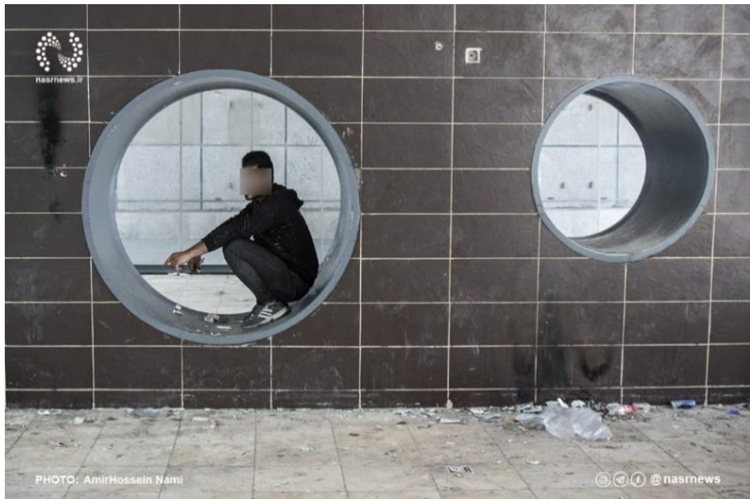
Figure 3.3: Beheshti Square turned into a ruin before being put into operation Sources: Yaz Echo. bit.ly/3Yw69VM (visited: February 19, 2023)
